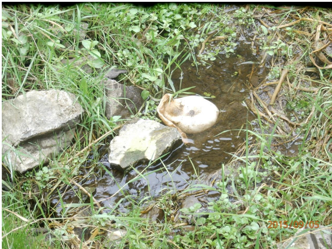
Swallow Hole No 1 adjacent to N15 Cotton installation on 05/09/2015
