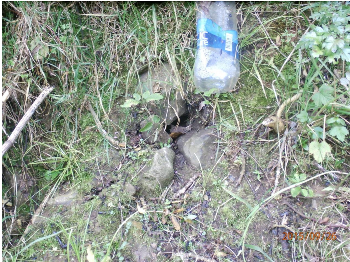
Dry Swallow Hole adjacent to SW No 1 (invert level 83.481mOD)
