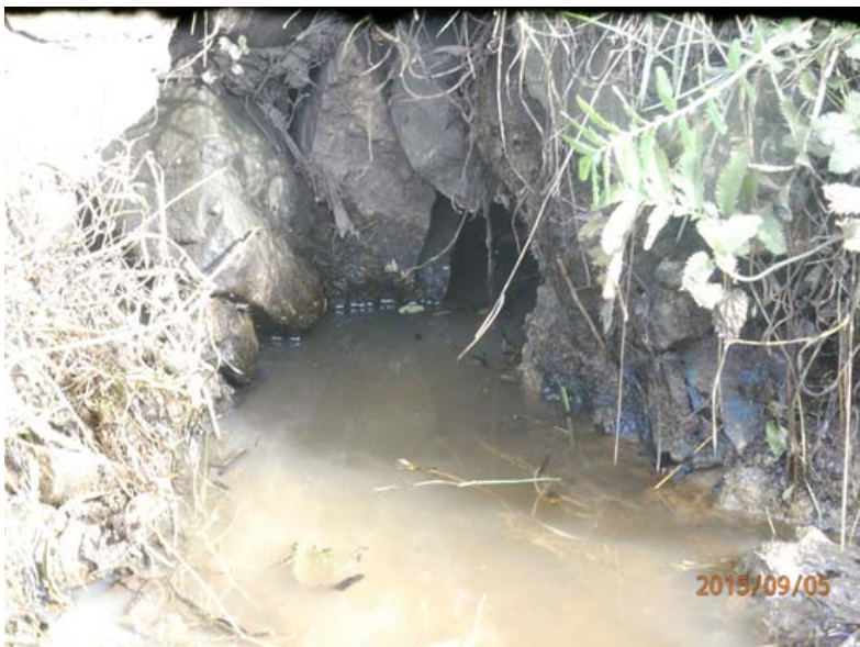
Active swallow hole, in ponded/flooded area, to the east of the N15 and east of the Gorman residence
