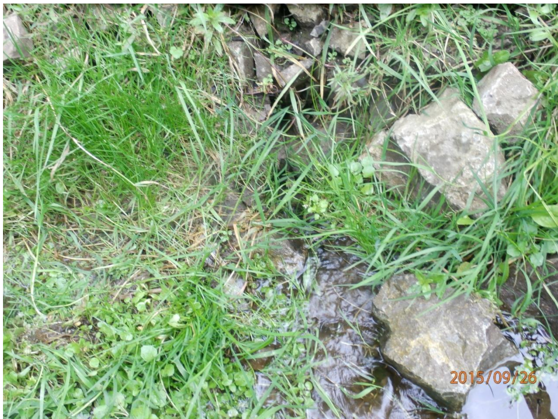
Swallow Hole No 1 (invert level 83.266mOD)
