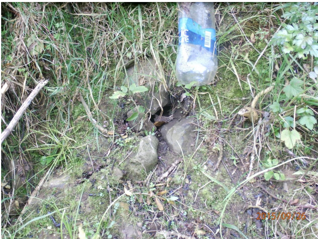
Swallow Hole adjacent to Swallow Hole No 1- Point ID 81 invert level 83.481mOD Swallow Hole dry on 26 th September 2015
